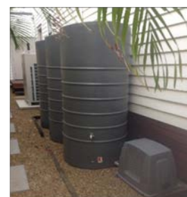
Water Tank / Pump
